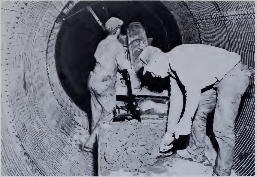
Figure 205. —Workmen shoveling mortar into a lining machine which will distribute it over the interior surface of a steel pipe. Reinforcement has been fastened to the surface to strengthen the lining. Normally, the lining is placed without reinforcement. P126-100-19.
